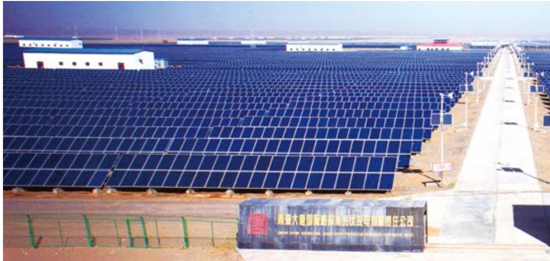
Qinghai Golmud Solar Photovoltaic Generation Company is the photovoltaic power plant with the largest installed capacity under China Datang Corporation.
